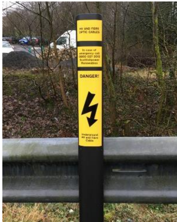
Figure 7. Typical Marker Post
